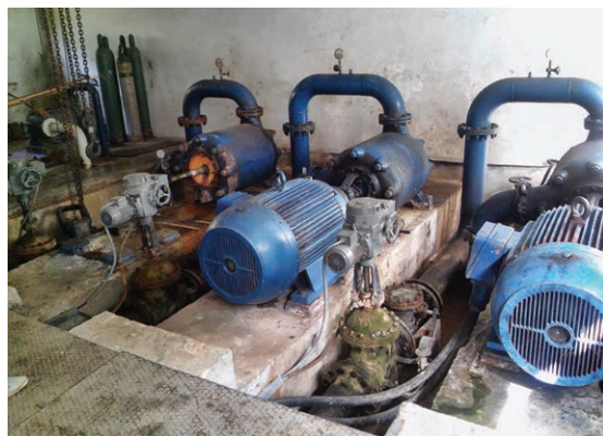
Hydro-mechanical equipment in pumping station Krupić (HEIS, 2015)
